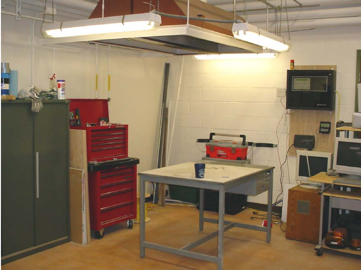
Small Fire Test Hood System.
