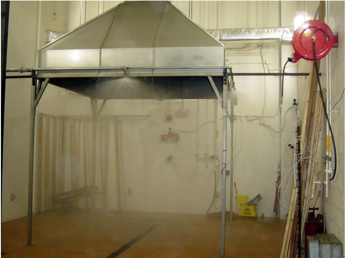
Large Hood system for one mega watt fires with deluge system flowing.
